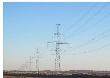
Figure 2. OT-GSK 220kV Transmission Tower
